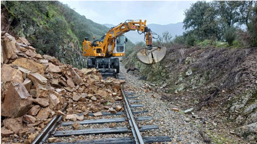
Figure 2 Rockslide identified by Sensonic DAS
