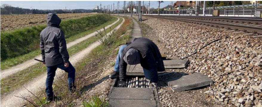
Figure 4 Cable theft on the railway.
