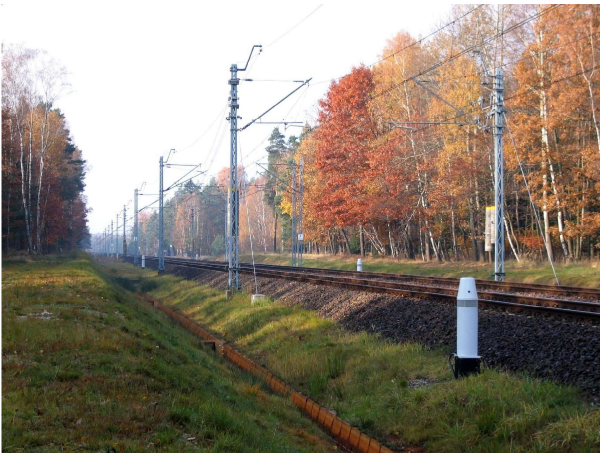
UOZ-1 Animal Protection Device on the railway line
