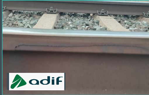
First critical defect identified by TCM application.
