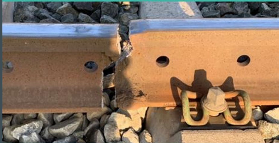
Broken rail / weld
